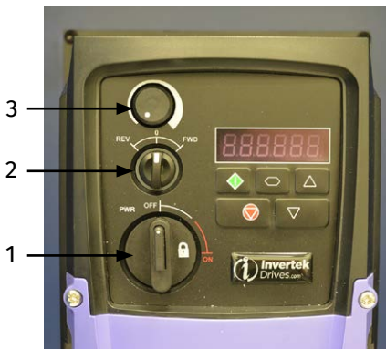
Fig. 8a Pump operation switches
